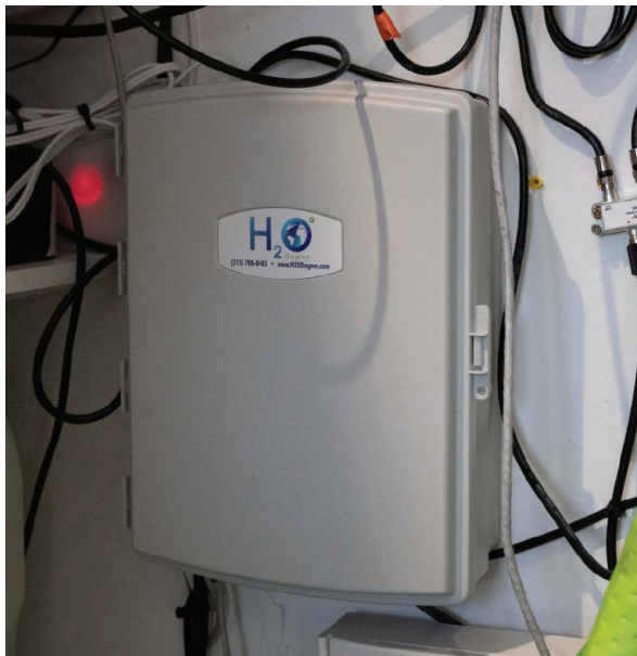
The MachineQ 8-channel indoor gateway is housed in an H2O Degree case within a utility closet in the apartment complex's centralized leasing office.
