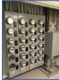
Figure 7. Electric submeters provided incentives for each tenant to conserve electricity at 360 State Street.
