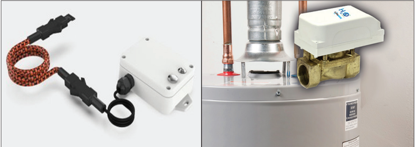
Figure 2. On-the-floor flood rope sensor (left) can detect flooding and pooling around a water heater and “tell” the smart valve (right) to shut off the water. Photo Courtesy: H2O Degree
